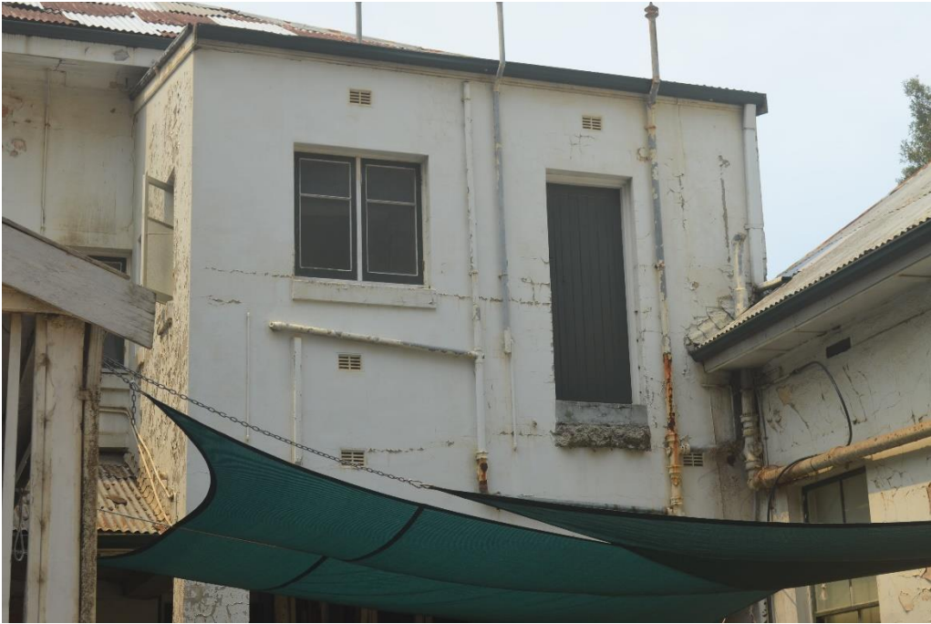
Figure 7: Existing external toilet block on first floor proposed to be demolished, viewed from southern side of site
